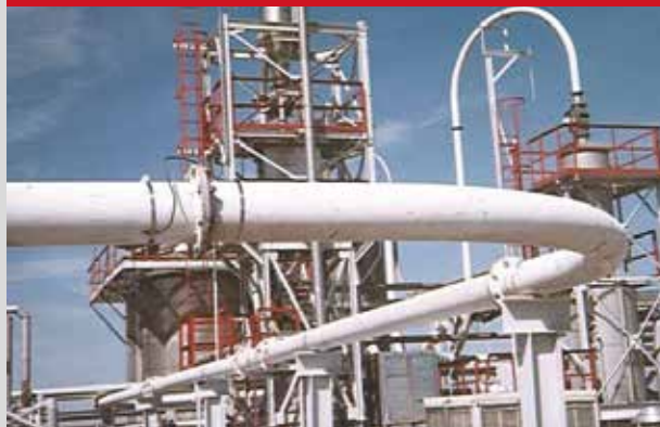
Fig. 10-6 Manufacturing Plant Utilizing Directionally Textured Pipe
